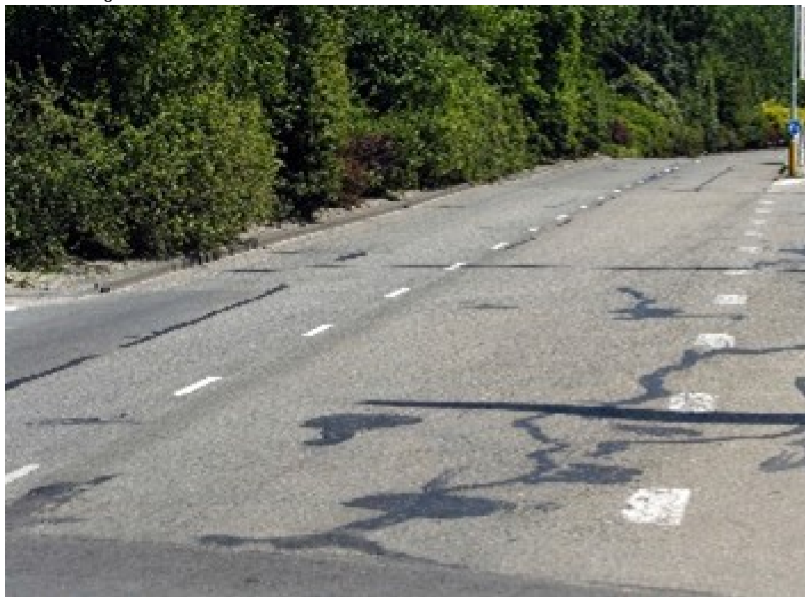
Scheurvorming asfalt (C)
