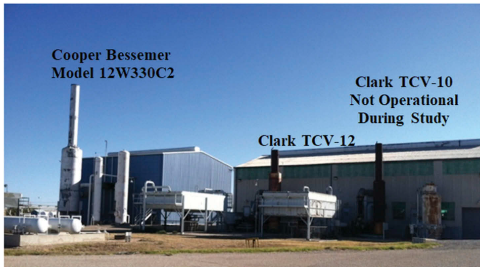
Figure 5.2 Sideview of the compressor units at the Balko compressor station (image copied from [20]). The boiler and the emergency generator were located farther to the left.
