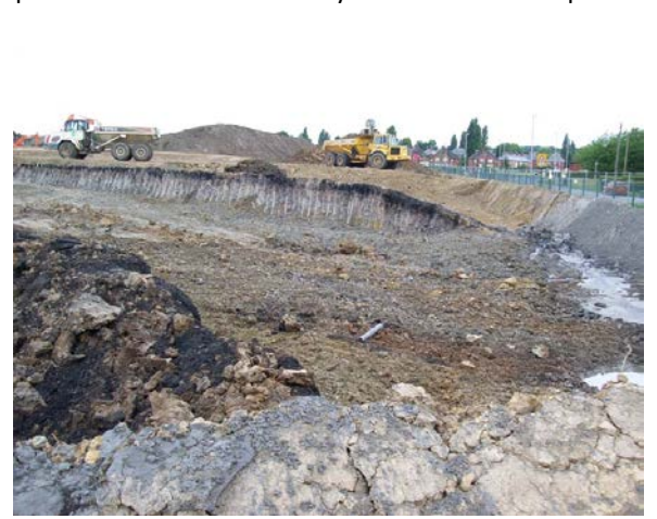
Outcrop of coal close to the surface which would be sterilised without prior extraction and has the potential to cause instability for surface development
