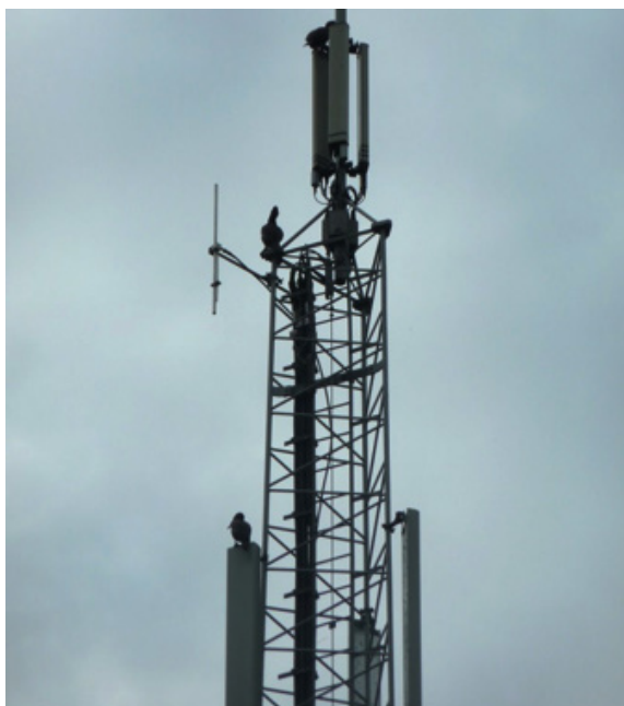
Illegale FM-antenne in mast mobiel netwerk
