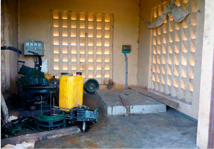
Collines, broken small piped water supply system
