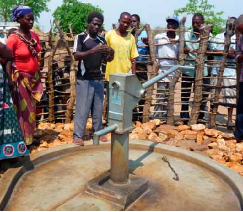
Borehole fitted with handpump
