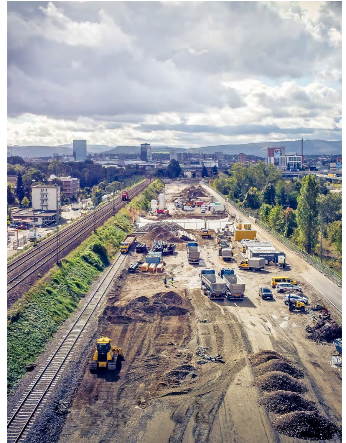
The access line to Basel Badischer Bahnhof under construction – this section is a crucial part of the 182 km long Karlsruhe-Basel rail link project.
