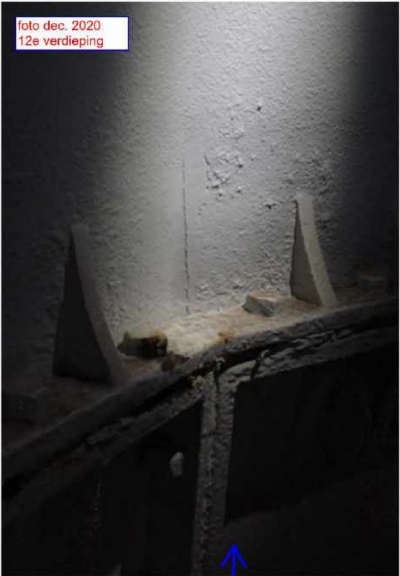
Verticale scheur in wand
